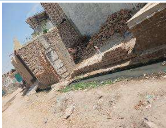
Open waste water drain
