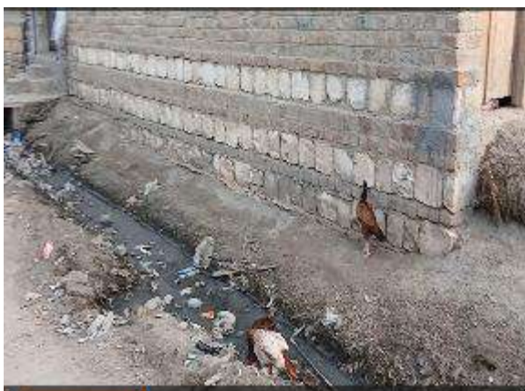
Poor wastewater drainage conditions are harming both livestock
